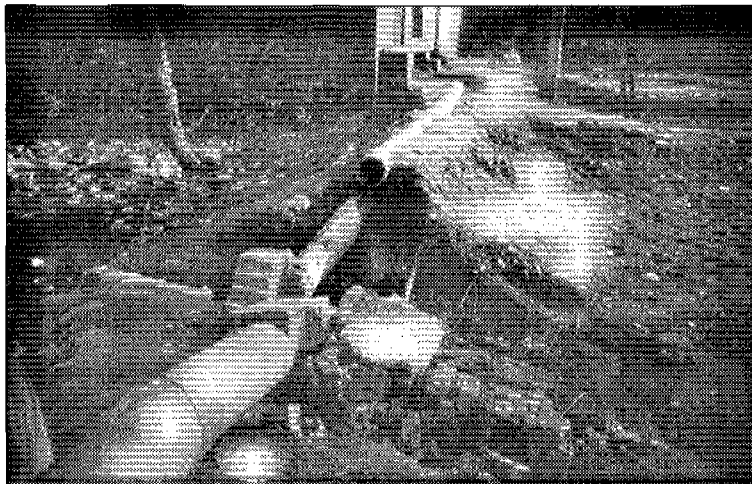
Figure 1.1 Community-built sewer in Lahore, Pakistan
