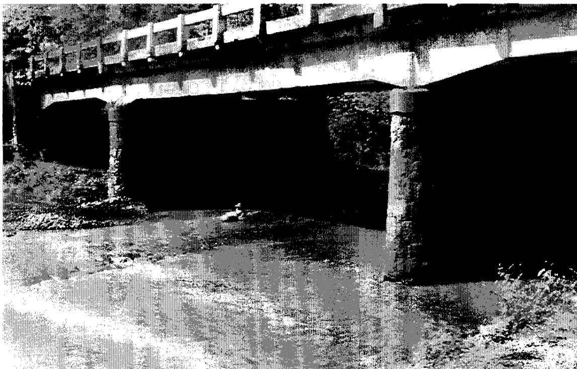
No. 3 The El Rosario River. Bridge on the Costal Highway (CA-2) with three openings. This river is the largest in the watershed.
