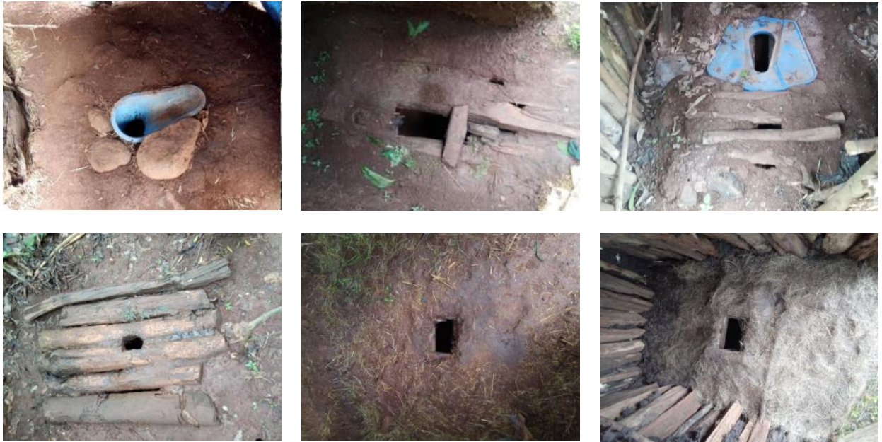
Figure 39: Examples of pit latrines defined as “unimproved” (i.e. with partly covered pits or floors that are not washable around the drophole such as mud/earth and wooden poles)
