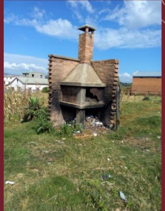
Broken incinerator at Saint Claire HC/Madagascar/Photo CRS Staff
