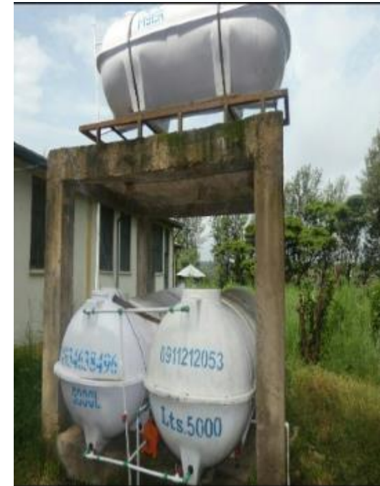
Water infrastructure after CCM, Wetet Abay HC/Photo CRS staff
