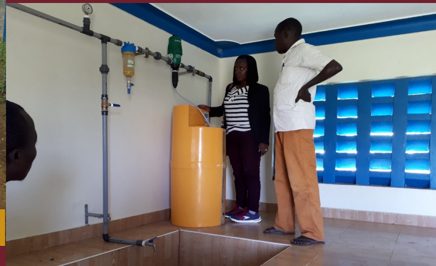
Treatment plant for a pumping system in Kapelebyong, 2018
