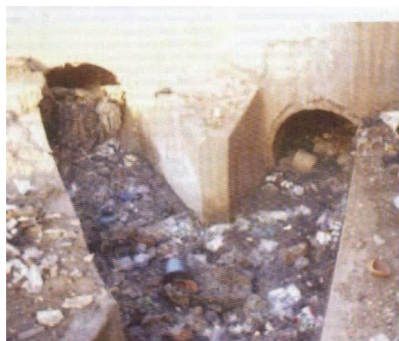
Figure 33: Solid waste clogging a drain
