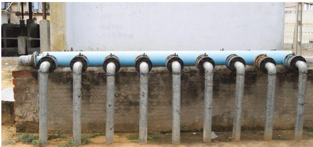
Photograph: Valve System in Sardhav
